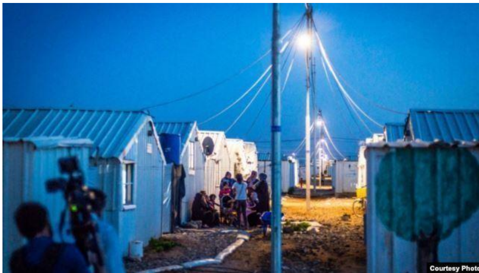
Figure 50. Solar streetlights, Zaatari (UNHCR,2019)
