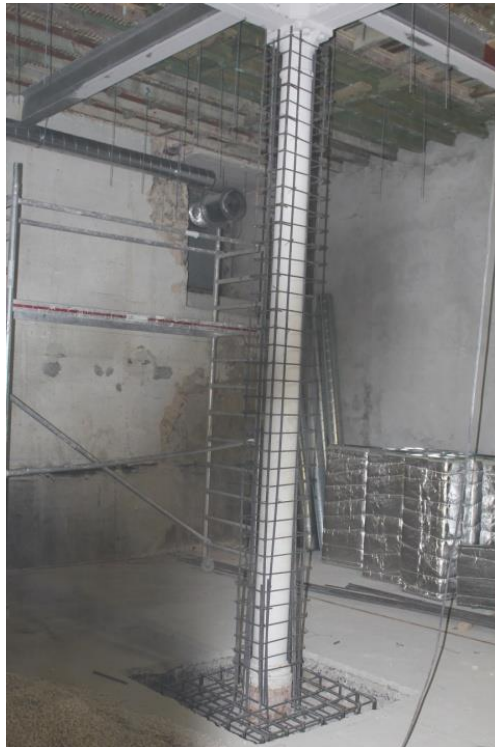
Figure 5 - Steel reinforcement of the wood structure in the basement ceiling. The enveloping of the iron cast column with concrete seems to us a bad solution, because it hides forever the history of the old structure and could be done, preferably in steel, easy to observe and easy to dismantle
