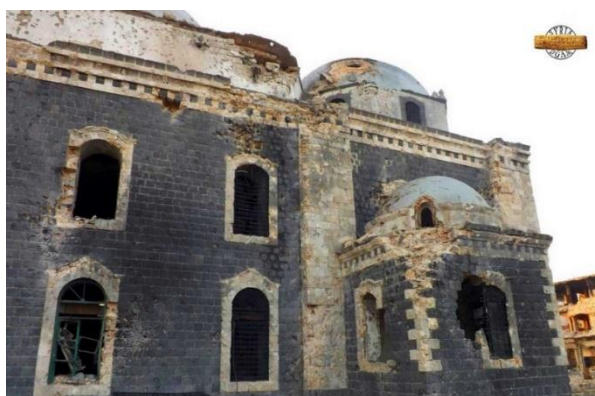
Fig. 60: Damages to Khalid Ibn Al-Walid mosque after the war.
