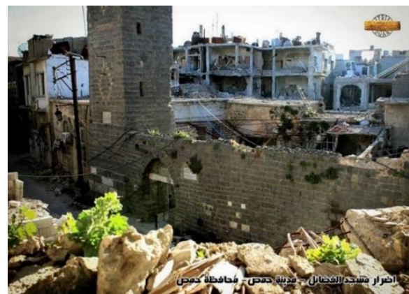
Fig.11: Neighbourhood in the old city of Homs, Abi Al-Fadael mosque, deterioration due to political conditions
