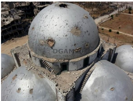
Fig. 58: Damages to the domes of Khalid Ibn Al-Walid mosque after the war.
