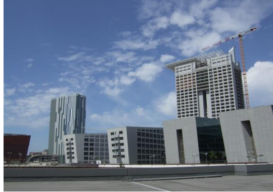
FIG. 7. Eur Sud – Castellaccio Central District. The two towers under construction (Franco Purini Architect and Studio Transit) [Photo: Antonio Cappuccitti and Alexandra Afrasinei]
