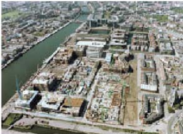
The extended 12-acre IFSC site in Dublin's Docklands. When complete, the site will employ 5,000 people, include 200 apartments, student and sheltered accommodation, shops, restaurants, a creche, a pub, a 4-star hotel and the NUI Docklands Campus.
